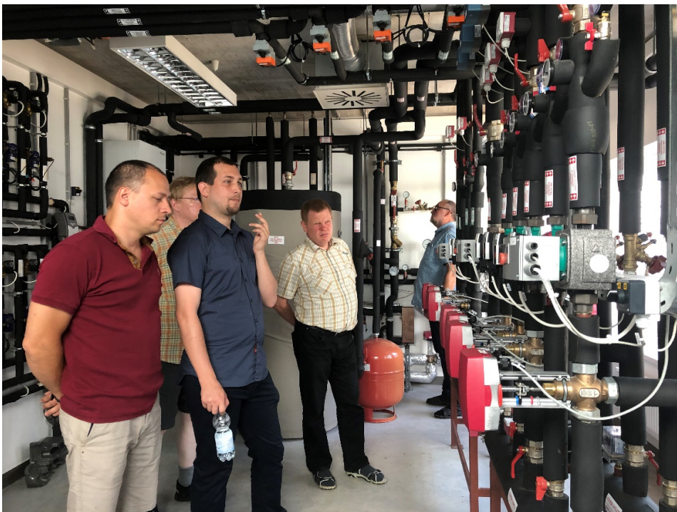
Inside the passive house ? Béla Bodó (left) is presenting the built in heating systems
